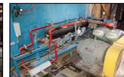
DRY KILN PUMPS
