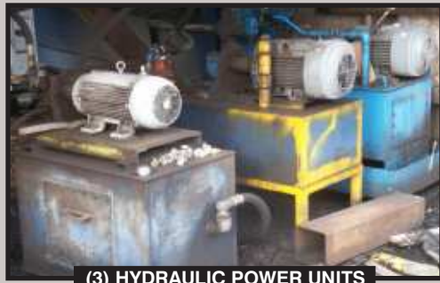
(3) HYDRAULIC POWER UNITS
