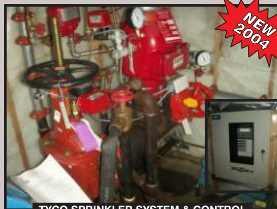
TYCO SPRINKLER SYSTEM & CONTROL
