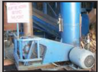
HOLMES 75HP BLOWER
