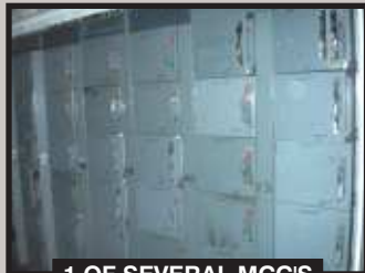
1 OF SEVERAL MCC'S
